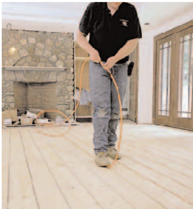
Figure 5. Once the panels are loosely attached to the floor, the tubing is “walked” into the grooves. If necessary, the tubing can be persuaded into place with a rubber-coated dead-blow hammer.
