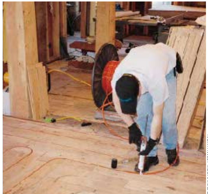
Figure 4. A continuous bead of silicone caulk is installed in each groove just before the tubing is installed.
