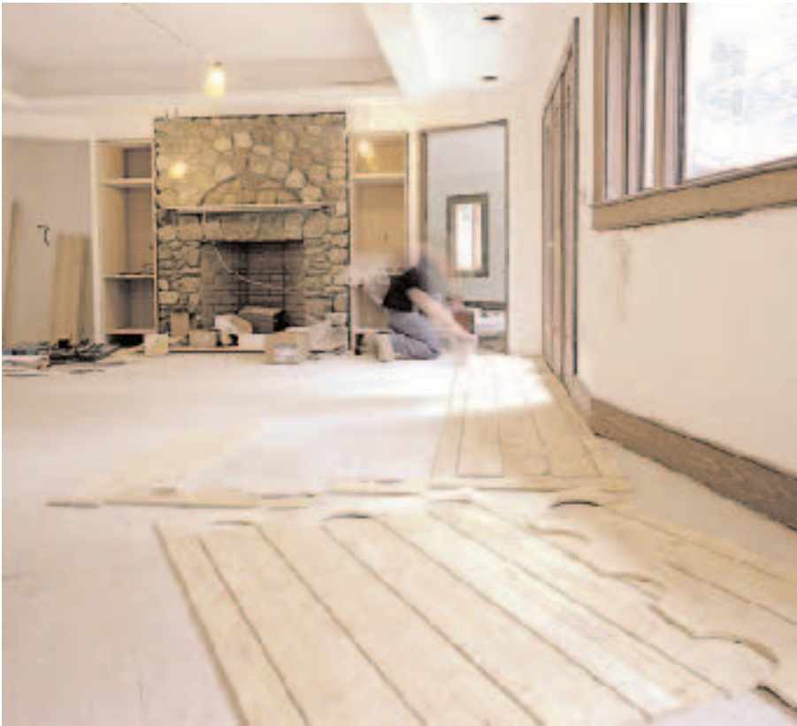
Figure 1. In this odd-shaped room, the author simplified the layout of the radiant flooring by dividing the space into separate rectangular areas, rather than having to cut and match angled sections of Climate Panel.
